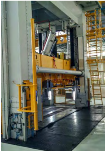
Automatic Swing Arm assembly duly interlocked with Slide Movement Photoelectric Guards & Two Hand Run Button Station for Operator Safety
