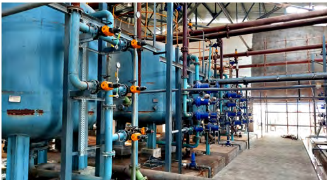
Complete Water and Wastewater Management Plant supplied to a Chemical Plant at Dahej, Gujarat, India
