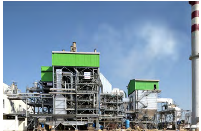
75 TPH Paddy Straw Fired Boiler supplied to an Independent Power Project in Haryana, India
