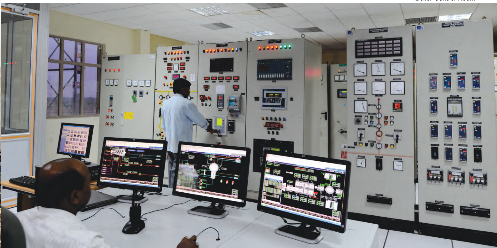
Boiler Control Room
