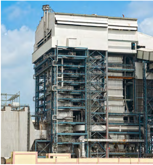
410 TPH Reheat type CFBC Boiler at Nirma Ltd., Bhavnagar (Gujarat) India for 70 MW Cogeneration Plant
