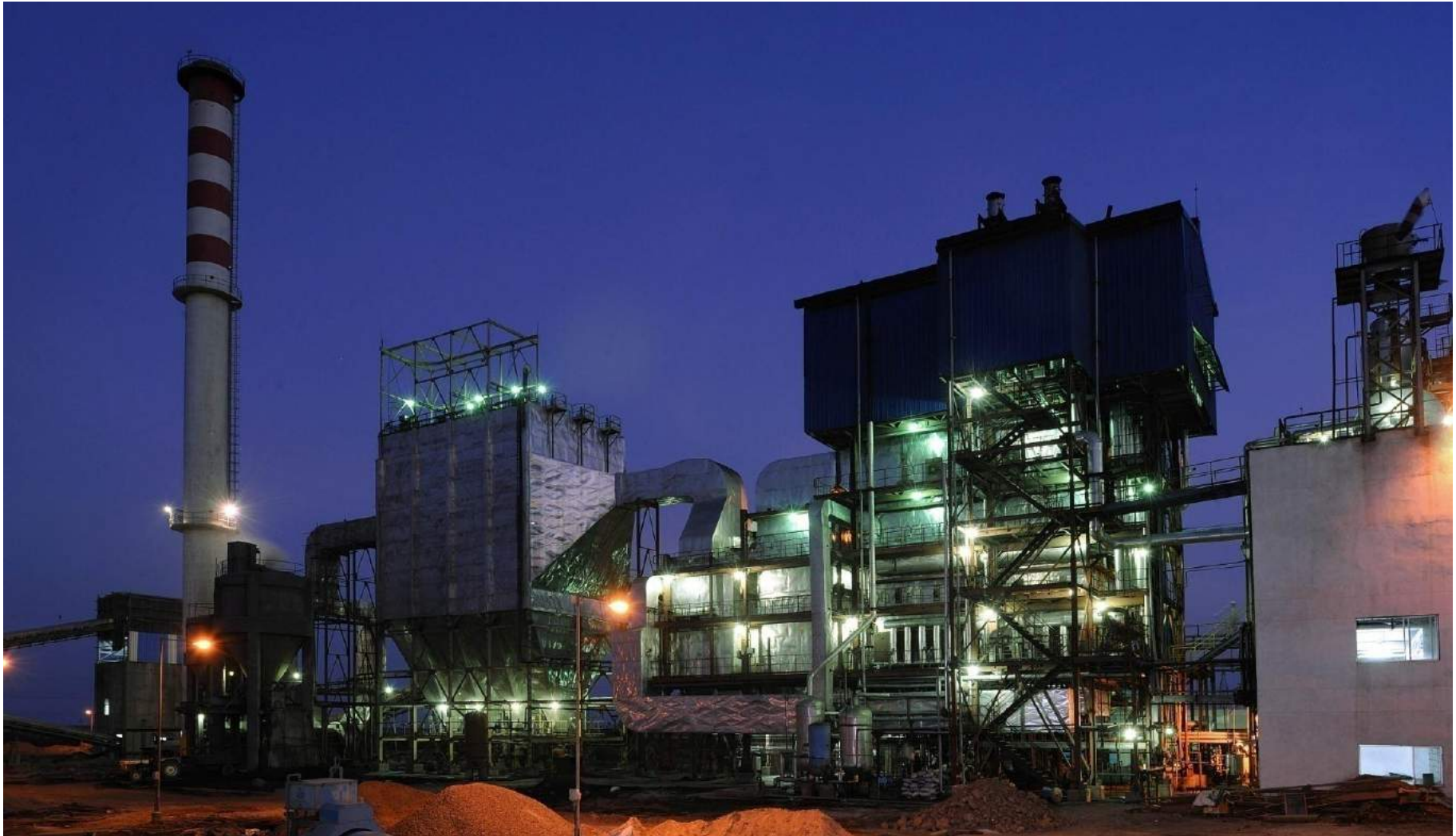
90 TPH, 67 kg/cm 2 (g), 485 ± 5 Deg.C AFBC Boiler
