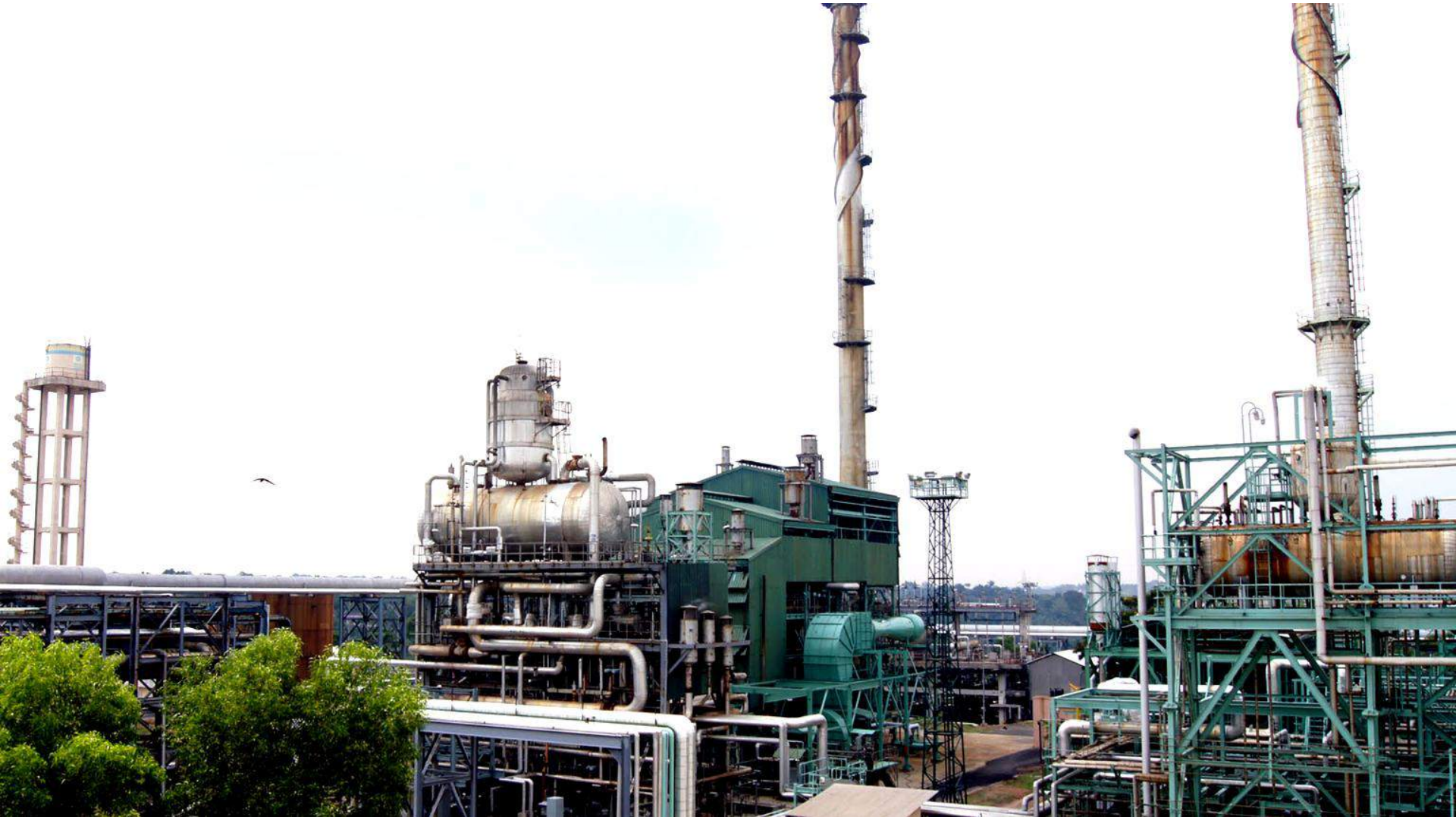
2 x 250 TPH Oil / Natural Gas Fired Boilers
