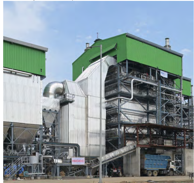
75 TPH, 94.2 ata, 540 Deg. C. Paddy Straw Fired Boiler at Sukhbir Agro, Kaithal, Haryana
