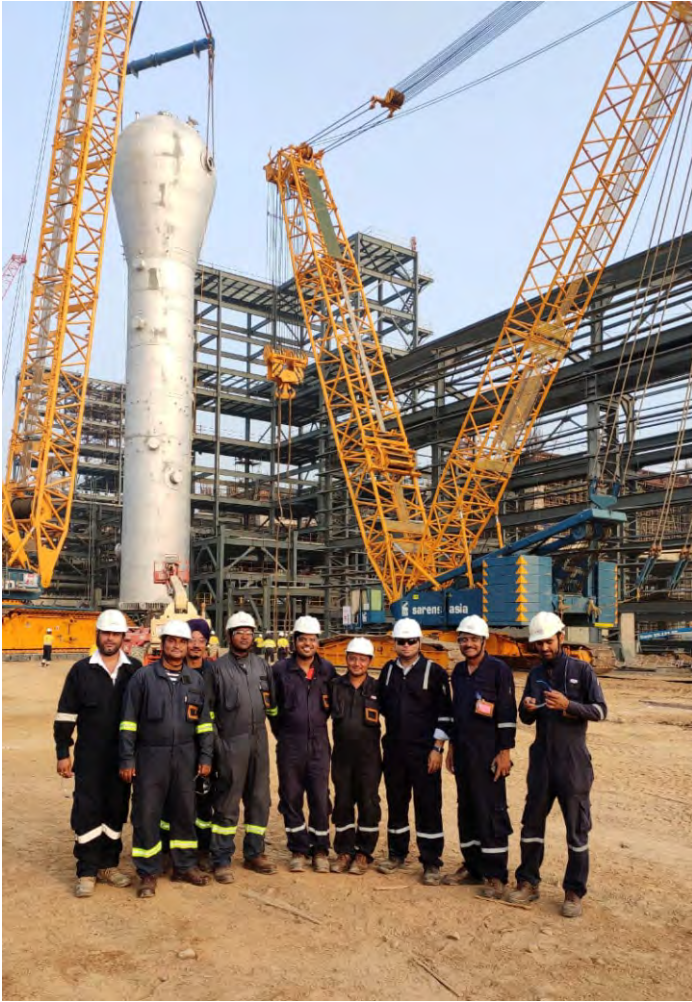
Site Fabricated Reactors
