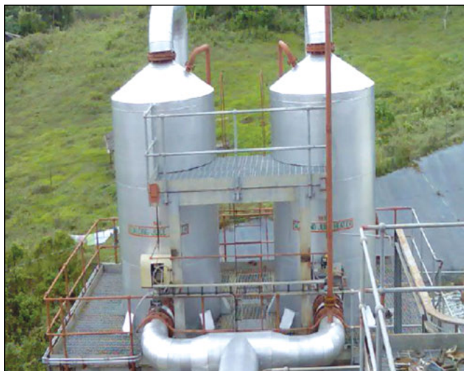
Figure 5. Battery of direct contact heaters
