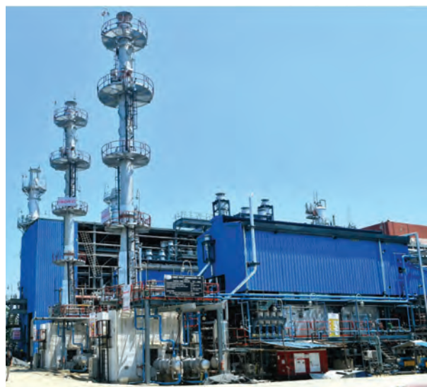
10 MW Gas Turbine based Power Plant supplied to a Petrochemicals Unit in Assam, India
