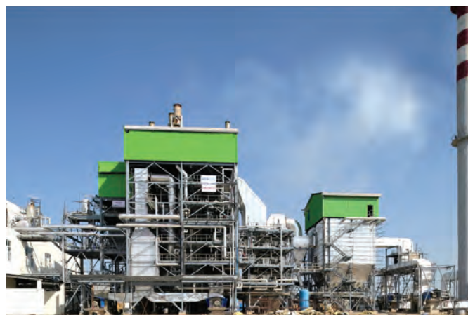
75 TPH Paddy Straw Fired Boiler supplied to an Independent Power Project in Haryana, India
