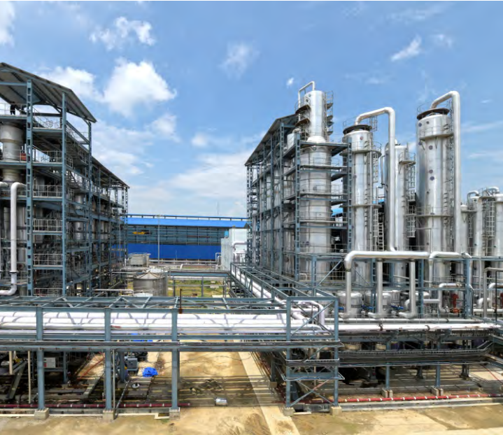
160 KLPD Distillery Plant at DCM Shriram Hariawan (U.P.), India
