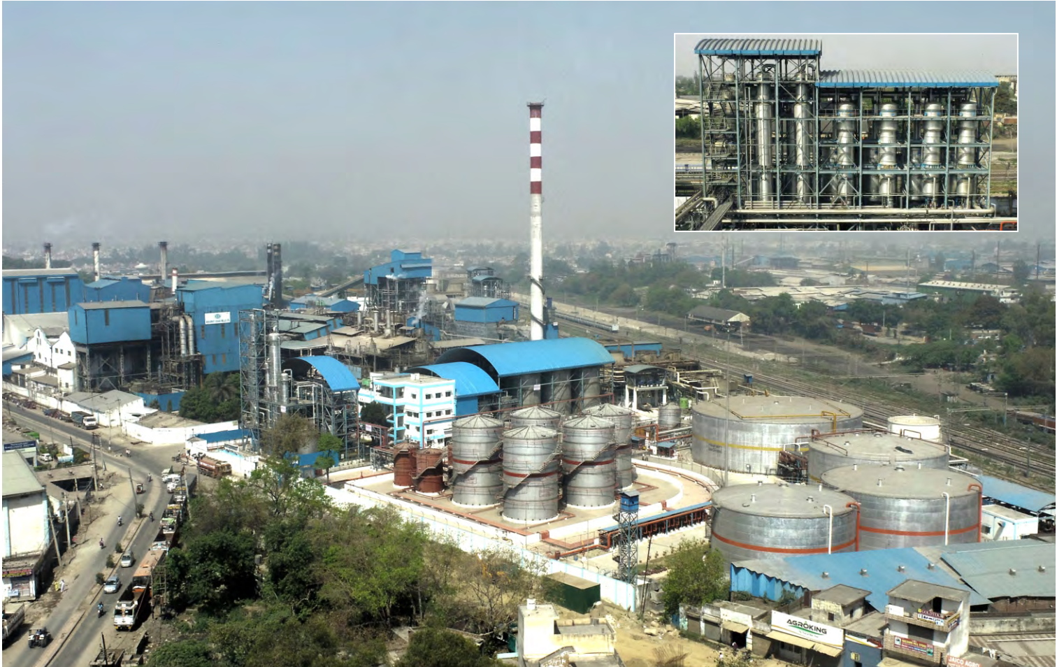
160 KLPD Multi-Feed Distillery with 48 TPH Slop Fired Incineration Boiler and 5.6 MW Power Plant on complete EPC basis including Civil Work at Saraswati Sugar Mills Ltd., Yamunanagar (Haryana)
