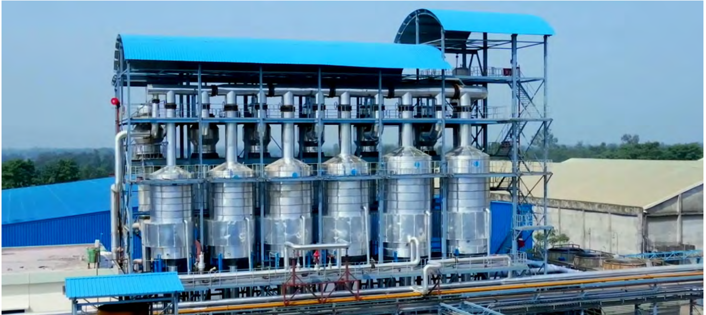
Spent Wash Evaporator System for 175 KLPD Ethanol Plant at Dwarikesh Sugar Ltd., India
