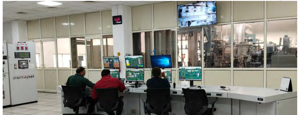
Centralised Control Room at a Distillery Plant
