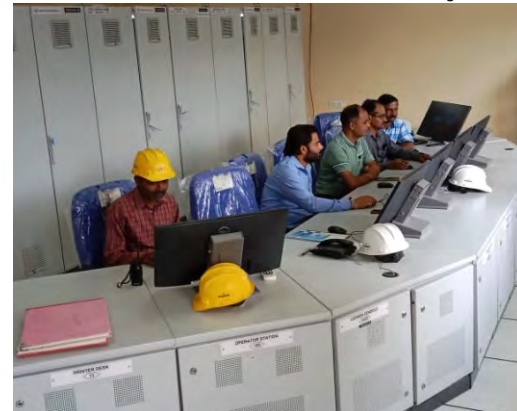
Centralised Control Room for a Sugar Plant
