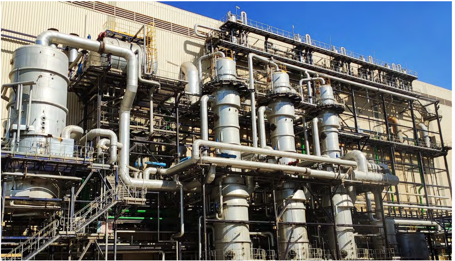
2500 TPD Standalone Refinery - Triple Effect Mill Concentrator Falling Film Evaporator at Durrah Advanced Development Company, Yanbu Port, Saudi Arabia
