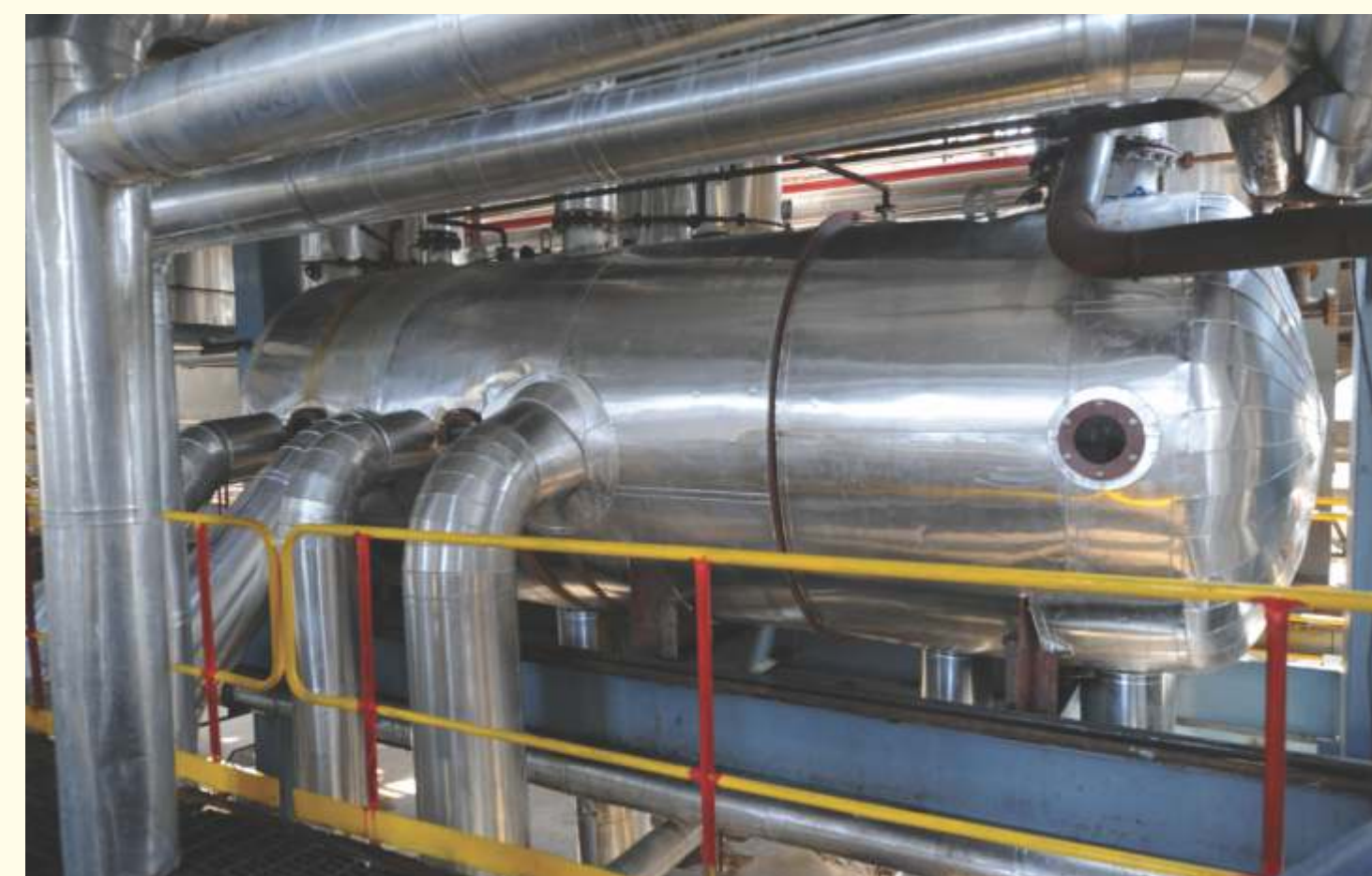
Condensate Flash Recovery Vessel
