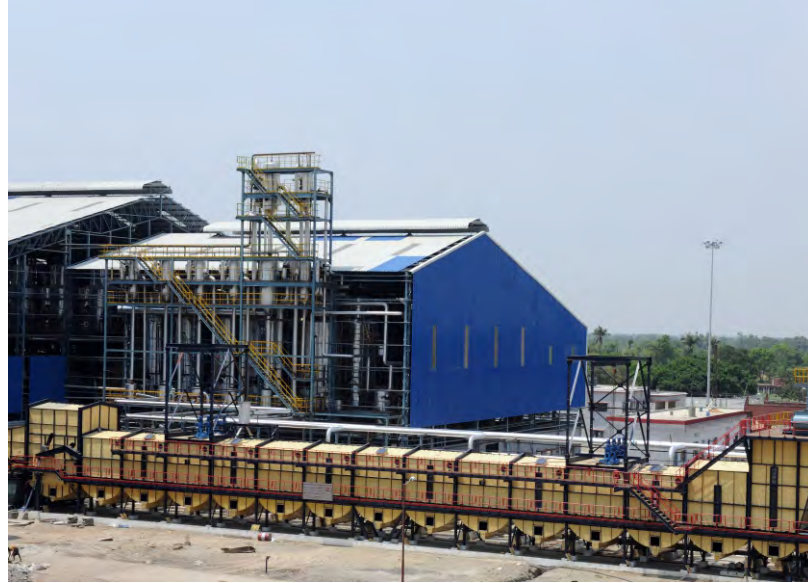
Chainless Cane Diffuser with Low Pressure Heating Module (LPHM) at HPCL Biofuels, Bihar, India
