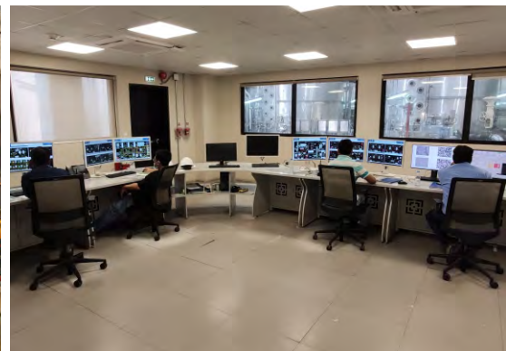
Centralised Control Room for a Sugar Plant
