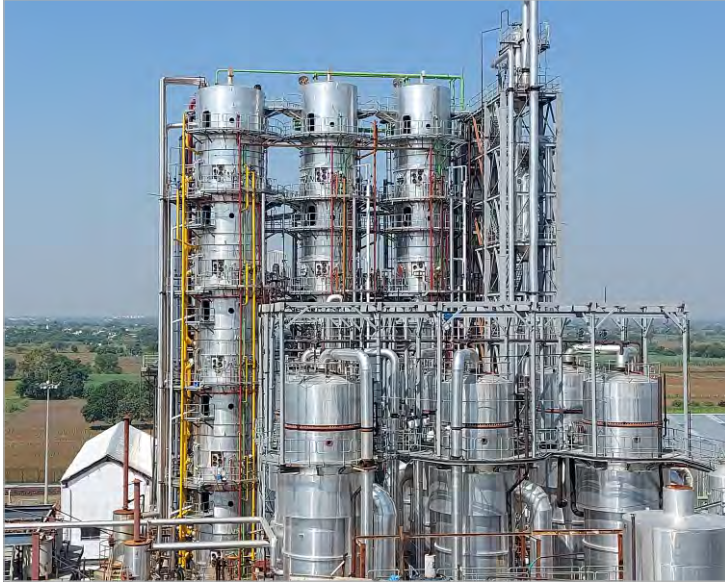
5000 TCD Sugar Plant-A/B/C Boiling Vertical Continuous Pan(VCP) at Twentyone Sugars Ltd., (Unit-1) Maharashtra, India
