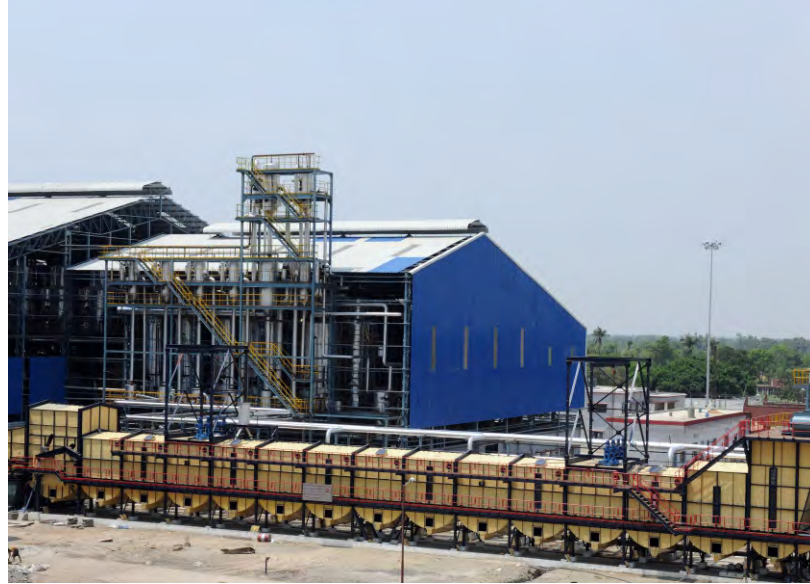
Chainless Cane Diffuser with Low Pressure Heating Module (LPHM) at HPCL Biofuels, Bihar, India
