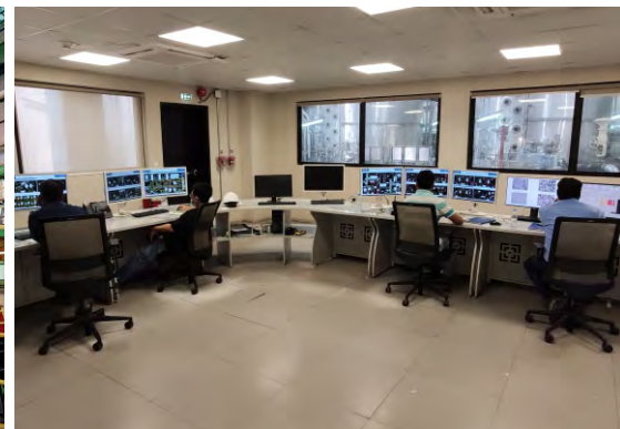
Centralised Control Room for a Sugar Plant
