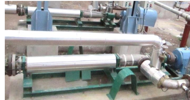
High pressure Vinasse Pump
