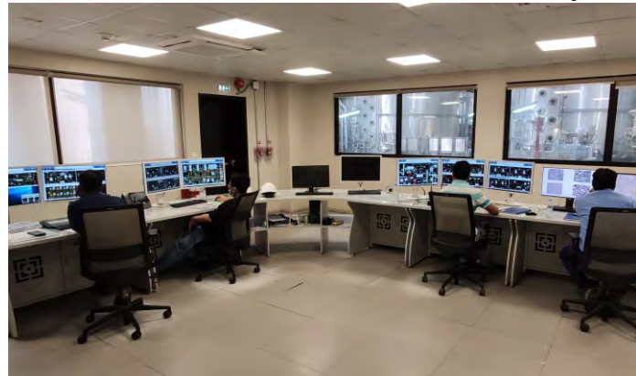
Centralised Control Room for a Sugar Plant
