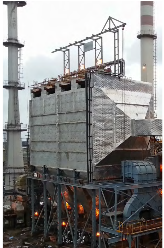
22 MW AFBC Power Plant at Gujarat Fluorochemicals Dahej, Gujarat
